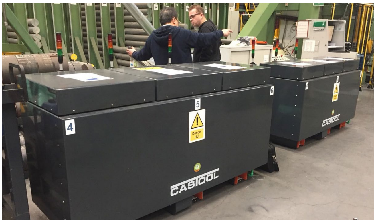
Installation of 2 TRC60 with Master Controller at MIFA - The Netherlands
