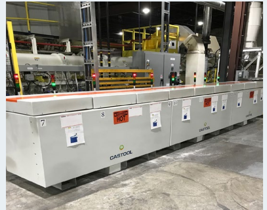
TCXi100 Install – Ontario, Canada
